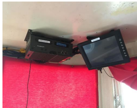
Computer processor and monitor installed on cabin ceiling.
