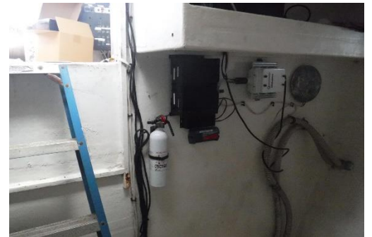
Processor installed in mid-cabin with Ethernet for cameras.
